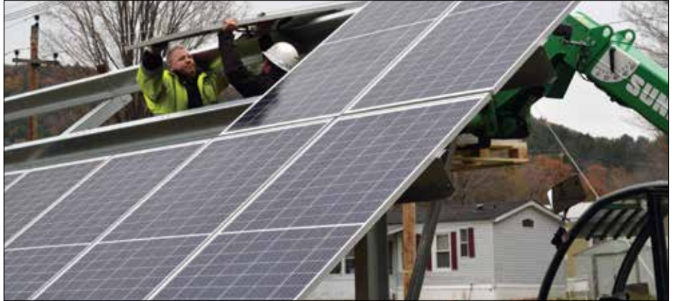
Workers install one of 384 solar panels in a 100-kilowatt array at Mascoma Meadows cooperative in Lebanon, N.H. Mascoma will be the first ROC in the Granite State to develop a revenue-generating solar project.
